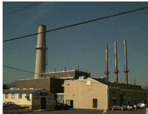
THE BUSCH COGENERATION PLANT (CAPACITY 14 MW), RUTGERS UNIVERSITY
